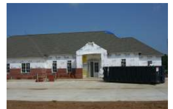
New Highland Road Office and Retail to take advantage of Baton Rouge's Green Light Plan
